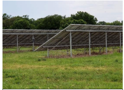
Example of a Solar Conversion System, Ground-mounted
